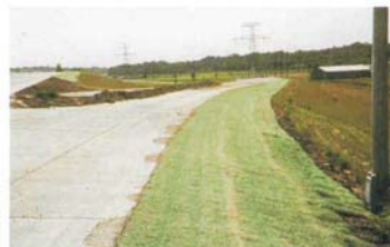
Curlex I QuickGRASS protects the shoulders from stormwater runoff before vegetation is established.
