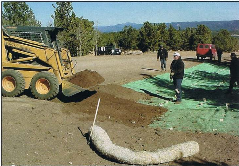
Soil loading of TRM to insure root reinforcement instead of stem reinforcement.
